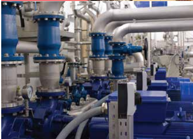
Plant equipment diagnosis and monitoring
