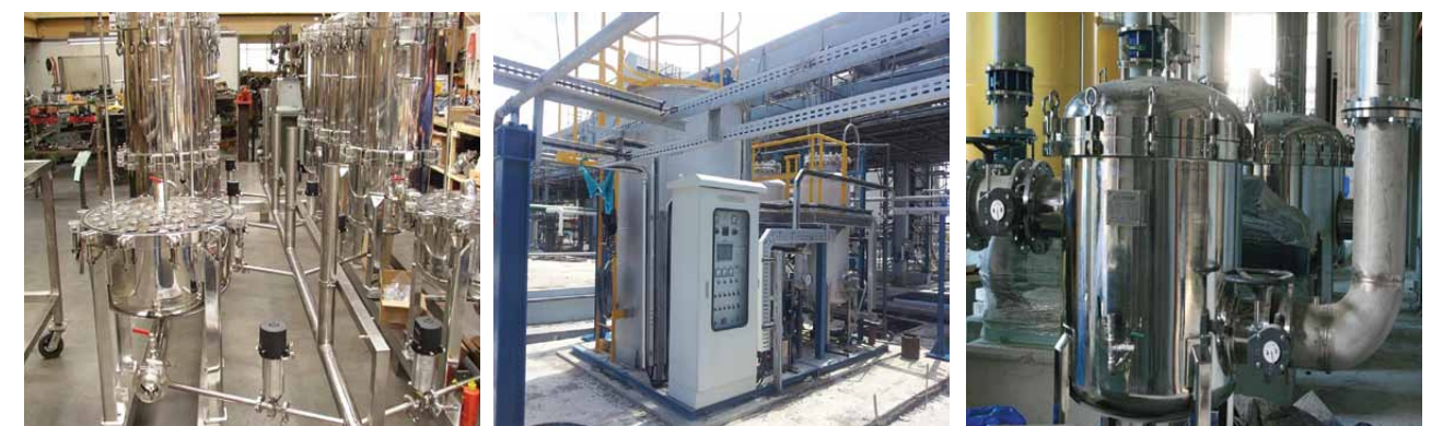
Water Treatment System
