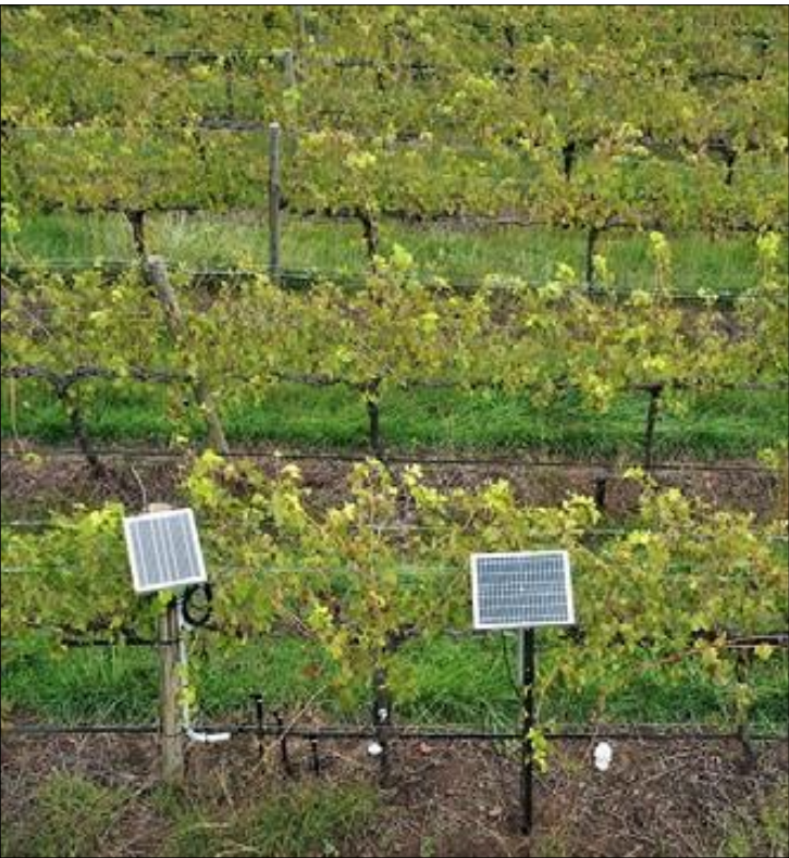
Vineyard Installation - MP406 Sensors Augered
